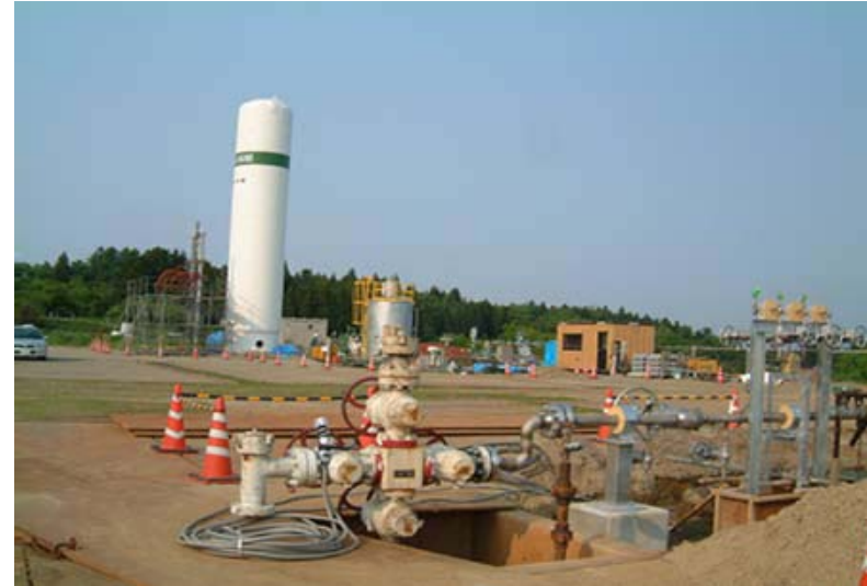
CO 2 injection facilities at Nagaoka, Japan
