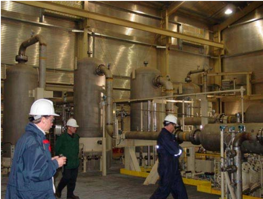
The CO 2 - compressor facility
