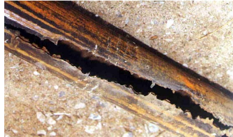
profile of tubing corrosion
