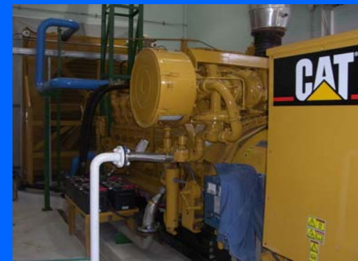
Electricity for Small Generator
